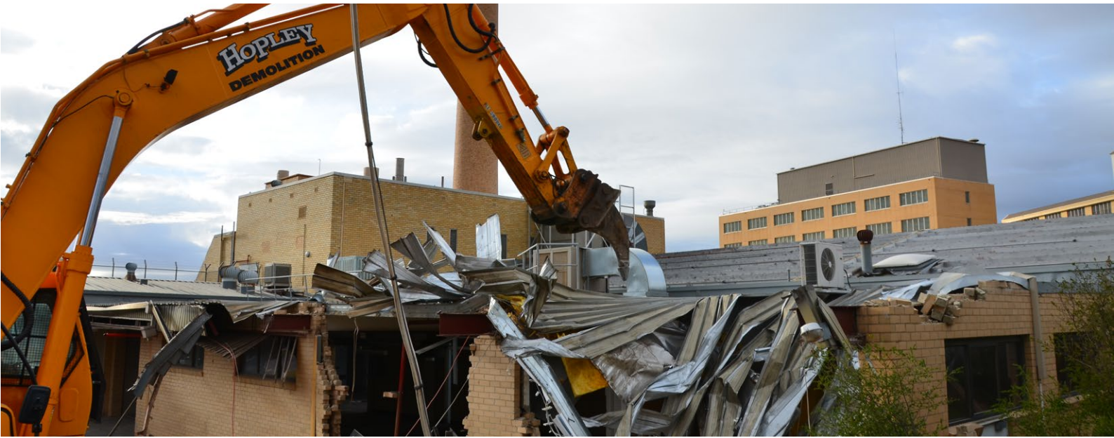
The former Loddon Linen service being demolished as part of preparatory works for the new Bendigo hospital.
