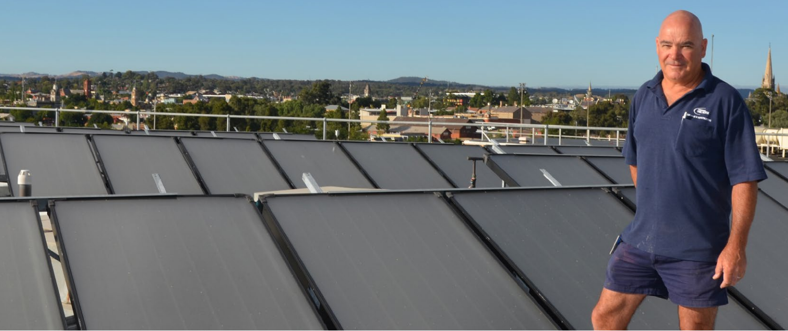
Brett Park, Plumber, with the solar hot water system on the roof of the Hyett building
