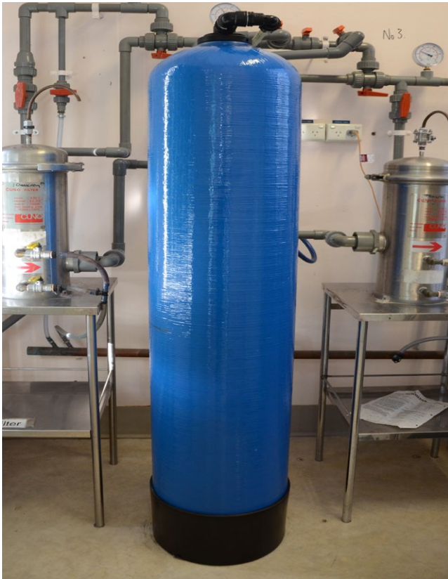
The reverse osmosis plant that treats drinking water to the standard required by dialysis services.
